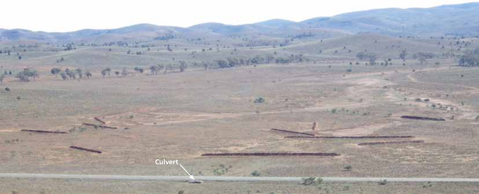
The view from Stokes Hill Lookout towards the soil banks developed on Willow Springs to re-direct water flow and spread it across the landscape. This will prevent further erosion as water moves through the road culverts. Brendan and Carmel plan to install a sign at the public lookout to describe the works undertaken.
